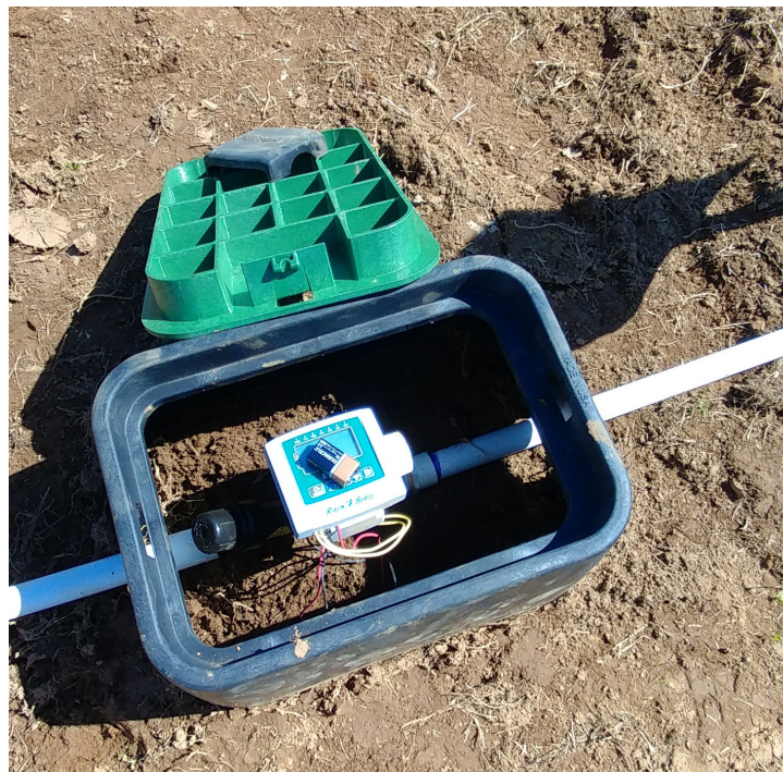
FIGURE 13. Irrigation box showing an automatic controller and one irrigation zone. Additional zones could be added if required. (Image source: Natalie Bumgarner)
